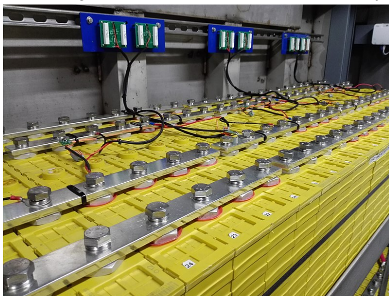
a large battery bank
